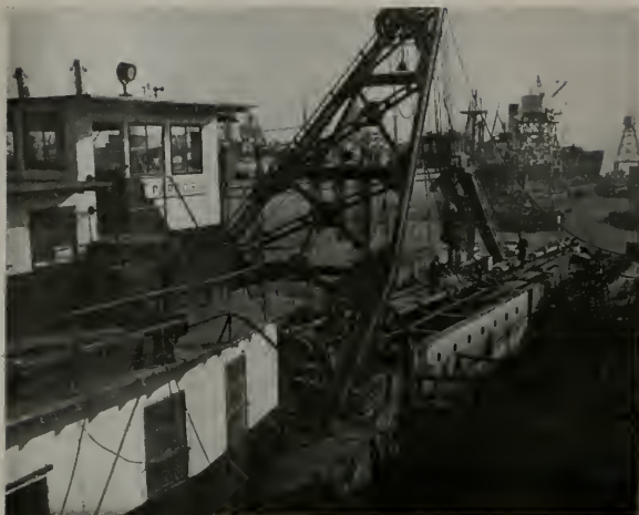
The hydraulic dredge Papoose, owned by the Hydraulic Dredging Company of Oakland, California, on the drydock at Bethlehem's San Francisco yard for re-installation of the 50-foot section in her dredging ladder in preparation for a contract to dredge for new berthing facilities at the San Francisco naval shipyard at Hunter's Point.
